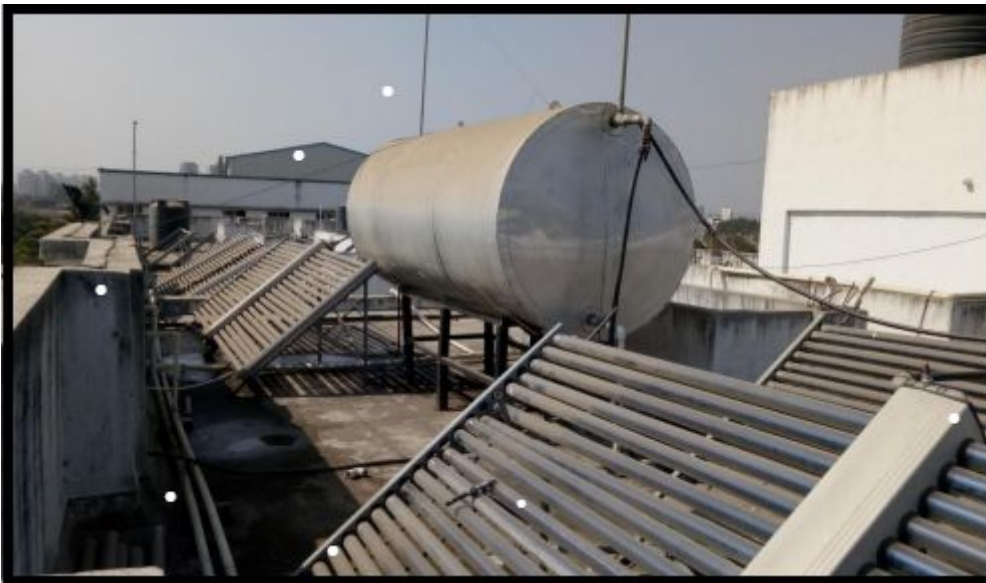
Solar Panel on Rooftop
